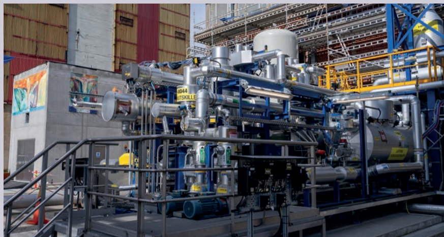
June 2024 saw Yara open a new renewable hydrogen plant in Herøya, Norway, the biggest hydrogen production facility of its kind in Europe.
