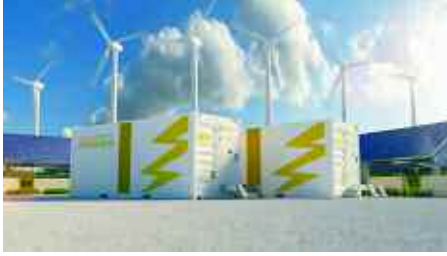
The big question about solar installations now relates to batteries.
