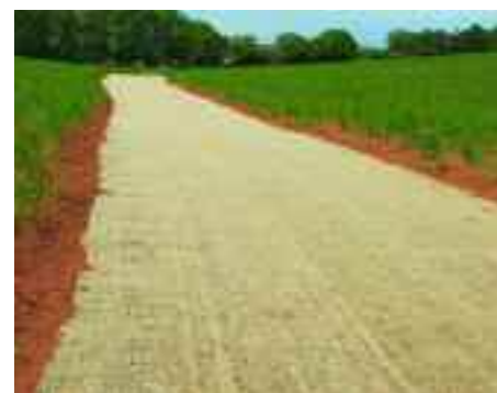
Grass waterway with jute geotextile to provide immediate protection from rainfall and runoff.
